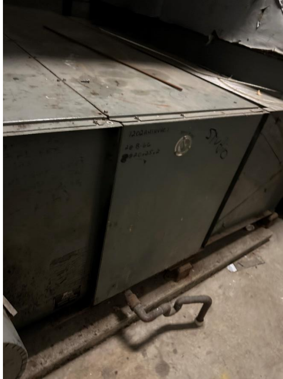
Upstairs AHU Serving Gym
