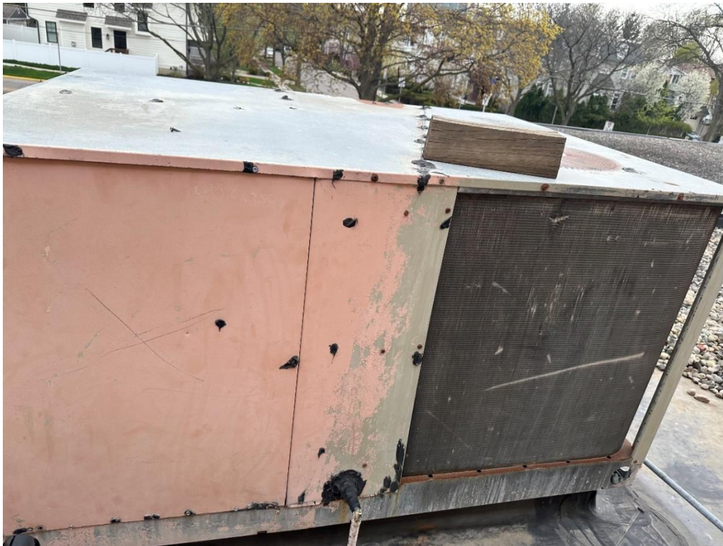
Wellness Center RTU
