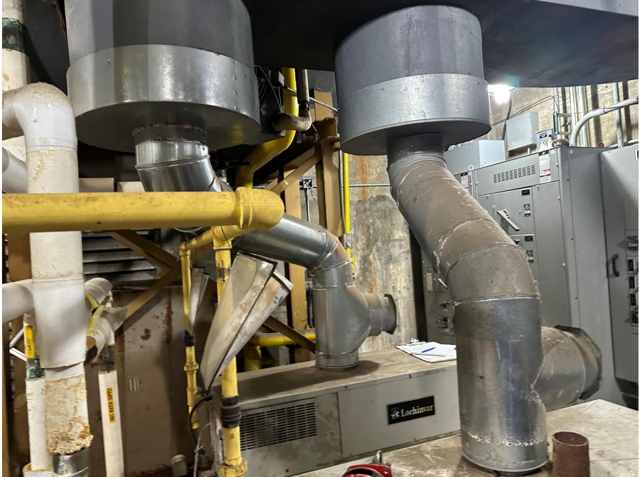
Water Heaters and Flue
