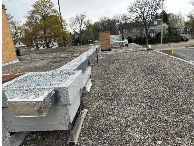
Weight Room RTU
