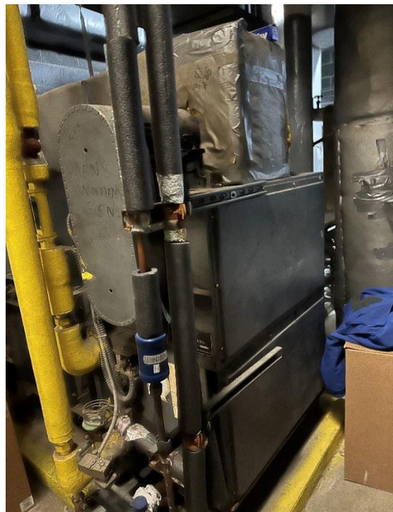
One Of Three Air Handling Units In Upstairs Mechanical Room
